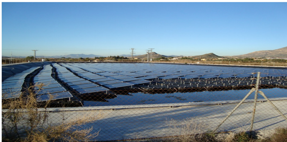
Figure 11. FPV system installed on the irrigation water reservoir in Spain [34].
