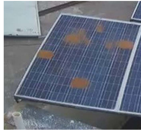
Figure 8. Partial shading due to soiling
